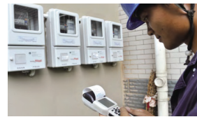
Wireless meter-reading system
